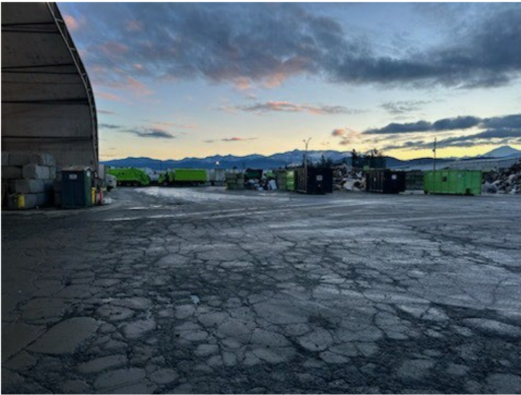
Photo 3. View of the significant asphalt cracking.
